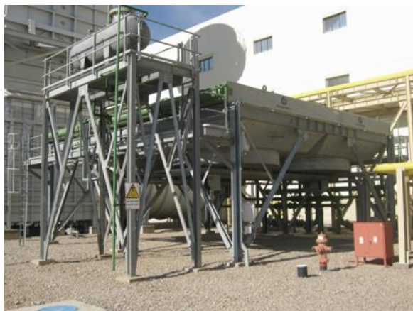
Figure 13. Set of fans and fin tubes of the V94.2-unit cooling system
